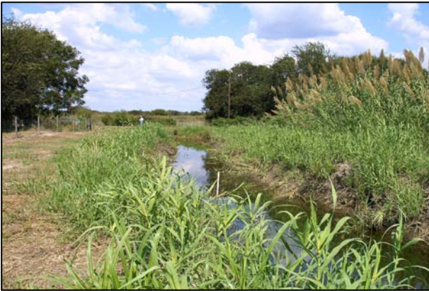
An overgrown section of the canal system
